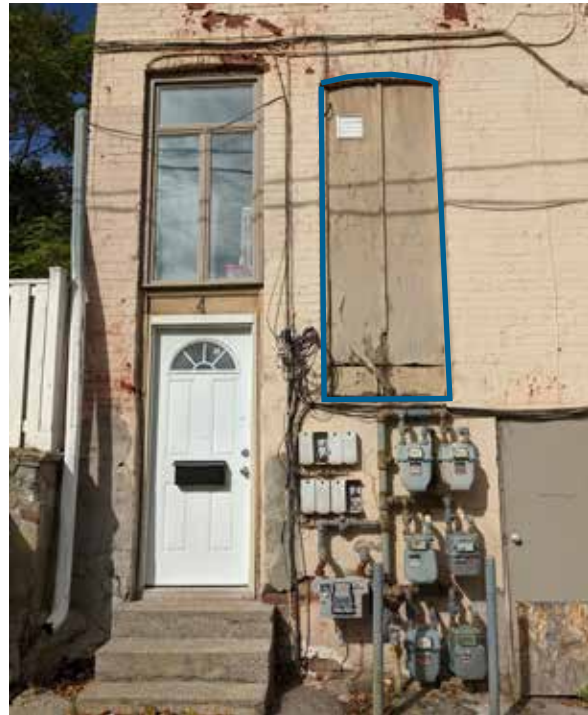
The original side door on Building A (outlined in blue) that floats above the first storey of Building A on the south elevation (ERA, 2021).
