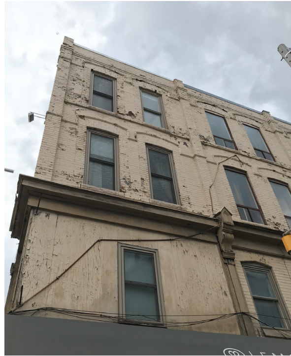
Defective condition of wood cornice (ERA, 2021).
