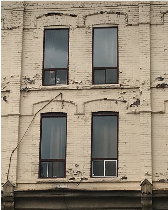
Peeling paint, deteriorated and damaged brickwork and masonry units (ERA, 2021).
