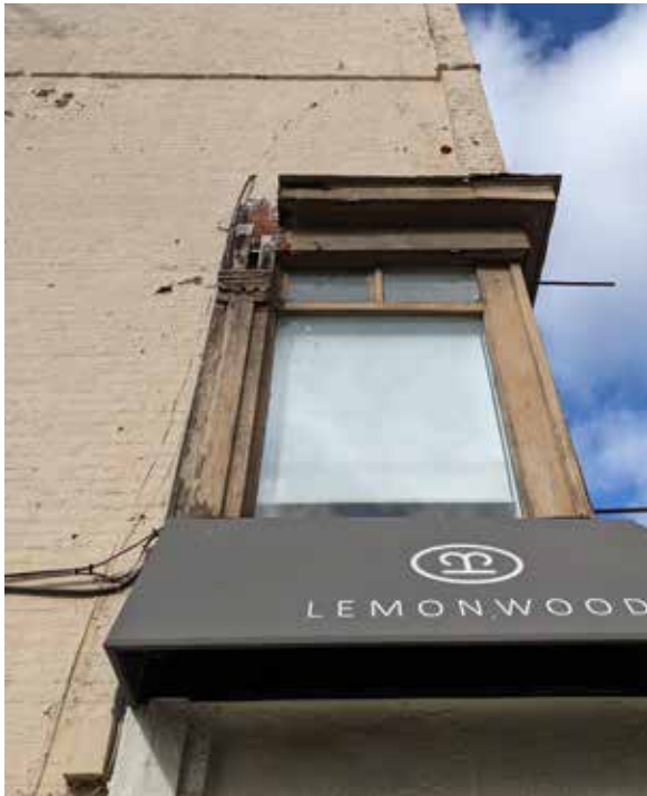
Remnant cornice on building A marking the top of the original retail bays, and the floating corner shop window with replacement glazing convey the historic grade line (ERA, 2021).
