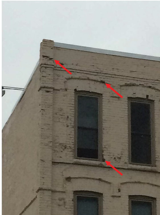
Photo #7: Typical view of deteriorated brick and mortar at 4 TH Floor on east elevation of Building 'A'.
