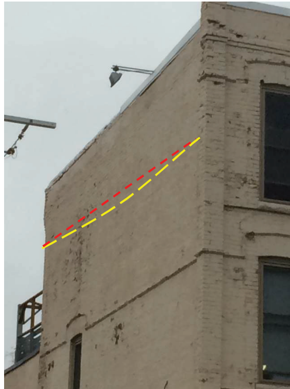
Photo #11: General view of south elevation of Building 'A'. At 4 TH Floor, the brick wall appeared to be visually bowed inwards approx. 6 to 8"
