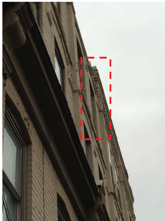
Photo #12: General view of parapet at Units 1202 and 1204. Parapets appear to be leaning inwards approx. 15 degrees.
