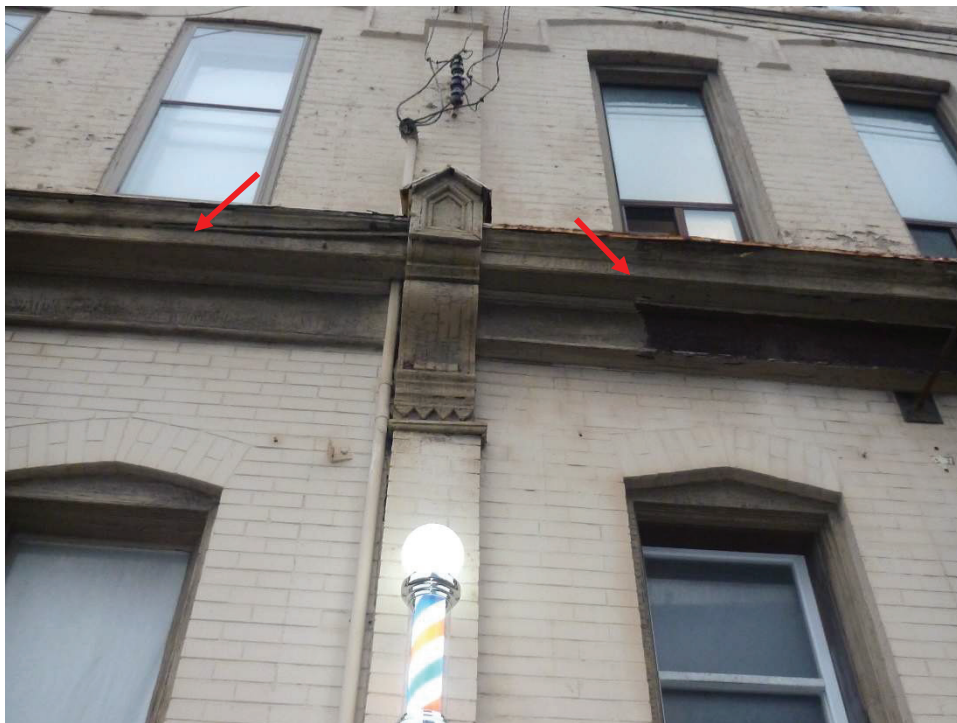
Photo #10: General view of existing wood cornice between 2 ND and 3 RD Floors at Building 'A'. Wood cornice appears to be undergoing significant deterioration.
