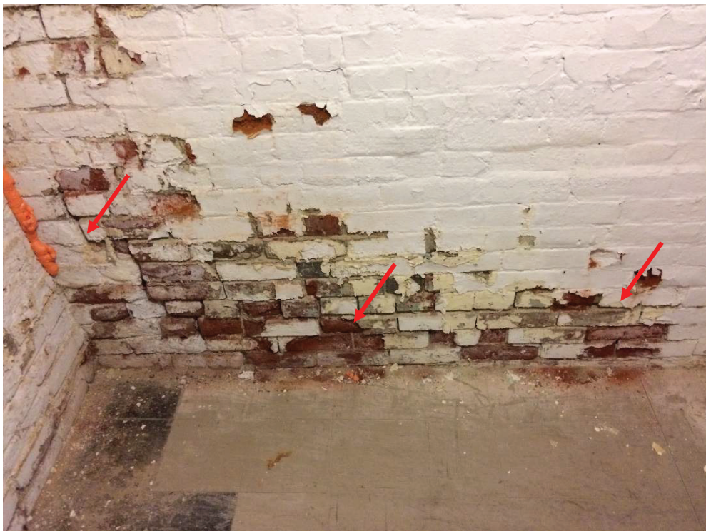
Photo #8: Typical view of deteriorated brick and mortar at base of exterior walls on interior side.
