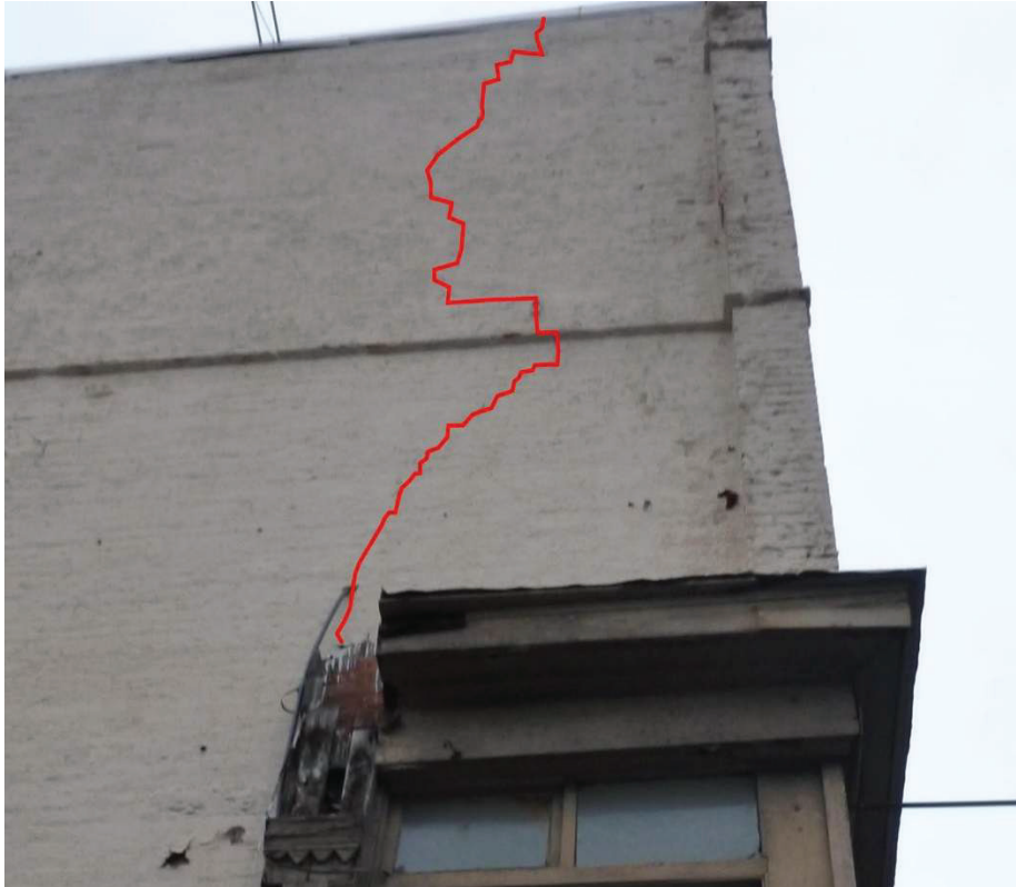
Photo #14: South elevation of southeast corner of Building 'A'. Enlarged view of step crack in brick wall.
